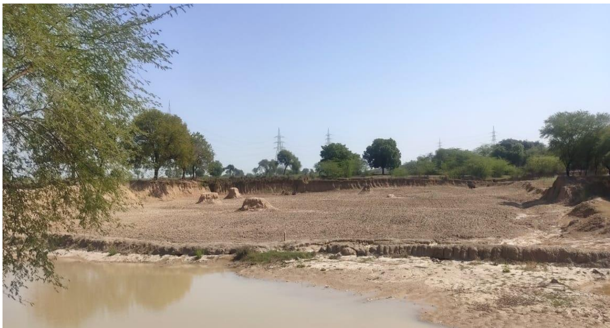
Figure 1. Soil removal for the construction of expressways in the Banda district of Bundelkhand (Source: Author)
