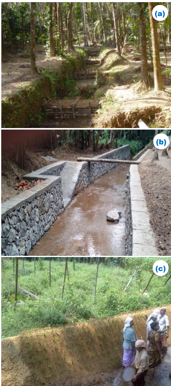
Figure 3: A view of (a) Log wood check dam (b) stream retaining wall (c) Geotextile walls
